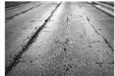
Multiple open cracks at center line, wheel paths and lane center.
